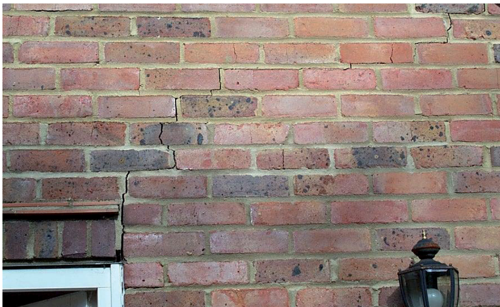
Figure 11 Damage to a property as a result of heaving clay soil beneath the ground beams where piled foundations have been used.
