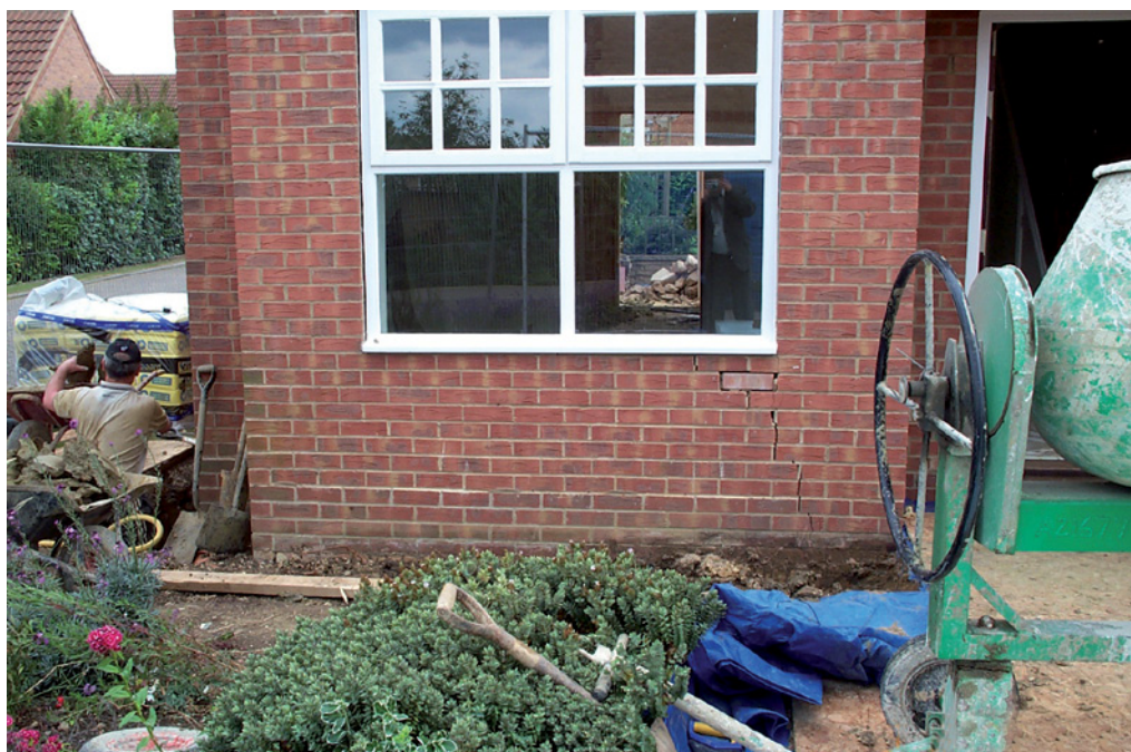
Figure 3 Example of damage, underpinning works are currently underway to prevent further movement occurring.
