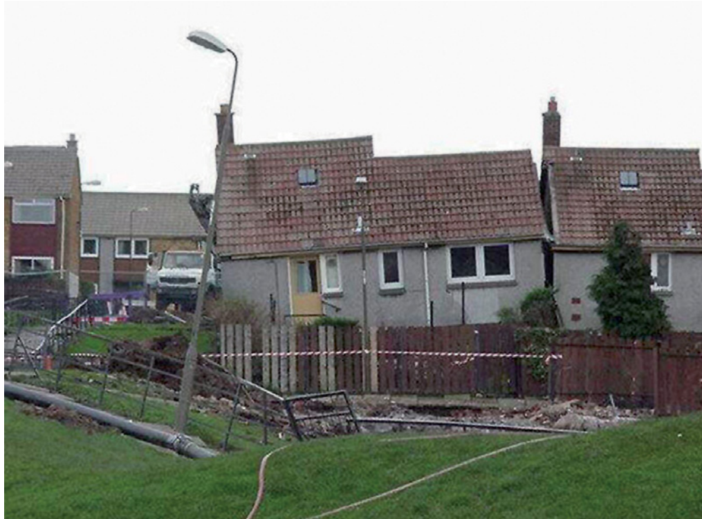
Figure 7 Subsidence associated with collapse of mining-related voids.
