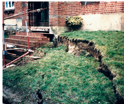
Figure 8 Damage due to landslip.
