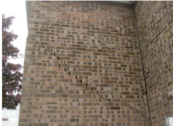
Figure 6: Extensive damage to a building with shallow trench fill foundations, caused by tree-related subsidence
