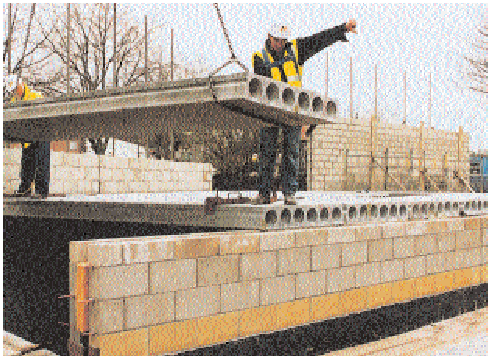
Precast hollowcore panels being installed on site (courtesy of Tarmac Topfloor Ltd)
