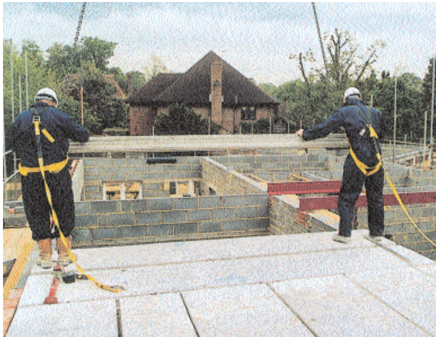
Safe, efficient erection of precast flooring (courtesy of Birchwood Concrete Products Ltd)
