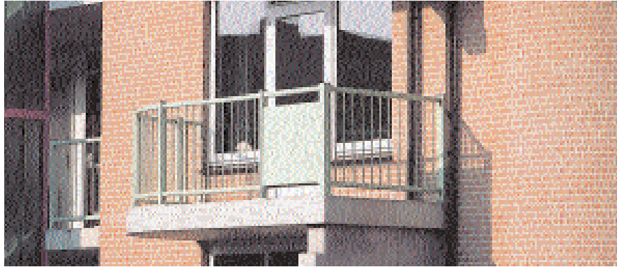
Simple precast balcony units add value to new apartments (courtesy of Belton/Bevlon)
