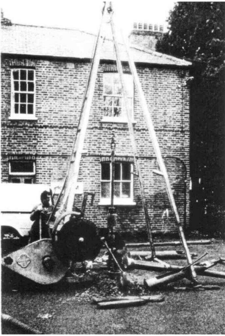
Figure 2.3 A typical shell boring rig at work on a housing site in Richmond, Surrey. Note the array of tools around the machine and the prepared undisturbed sampling tool in the background.
