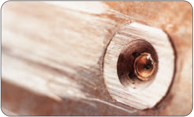
Figure 25 - Mode of Failure - Alignment
