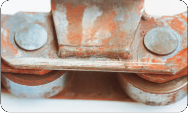
Figure 23 - Mode of Failure - Alignment
