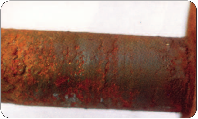
Figure 28 - Mode of Failure - Corrosion at High Temp
