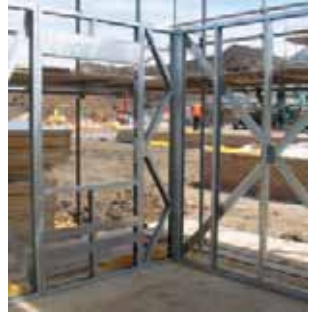
Open steel frame panels
