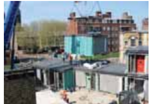
Flats being constructed with volumetric units – all the units shown were placed in one day
